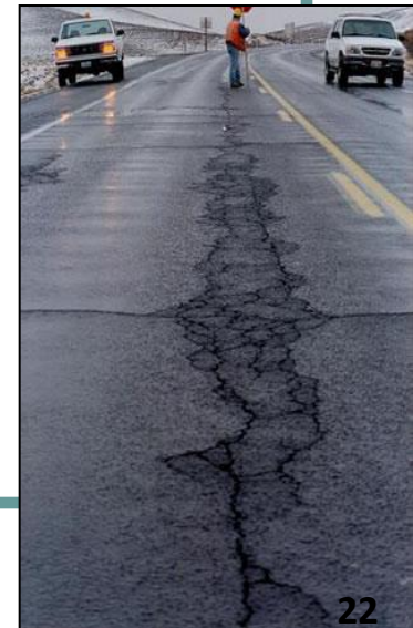
Fatigue cracking caused by stripping
