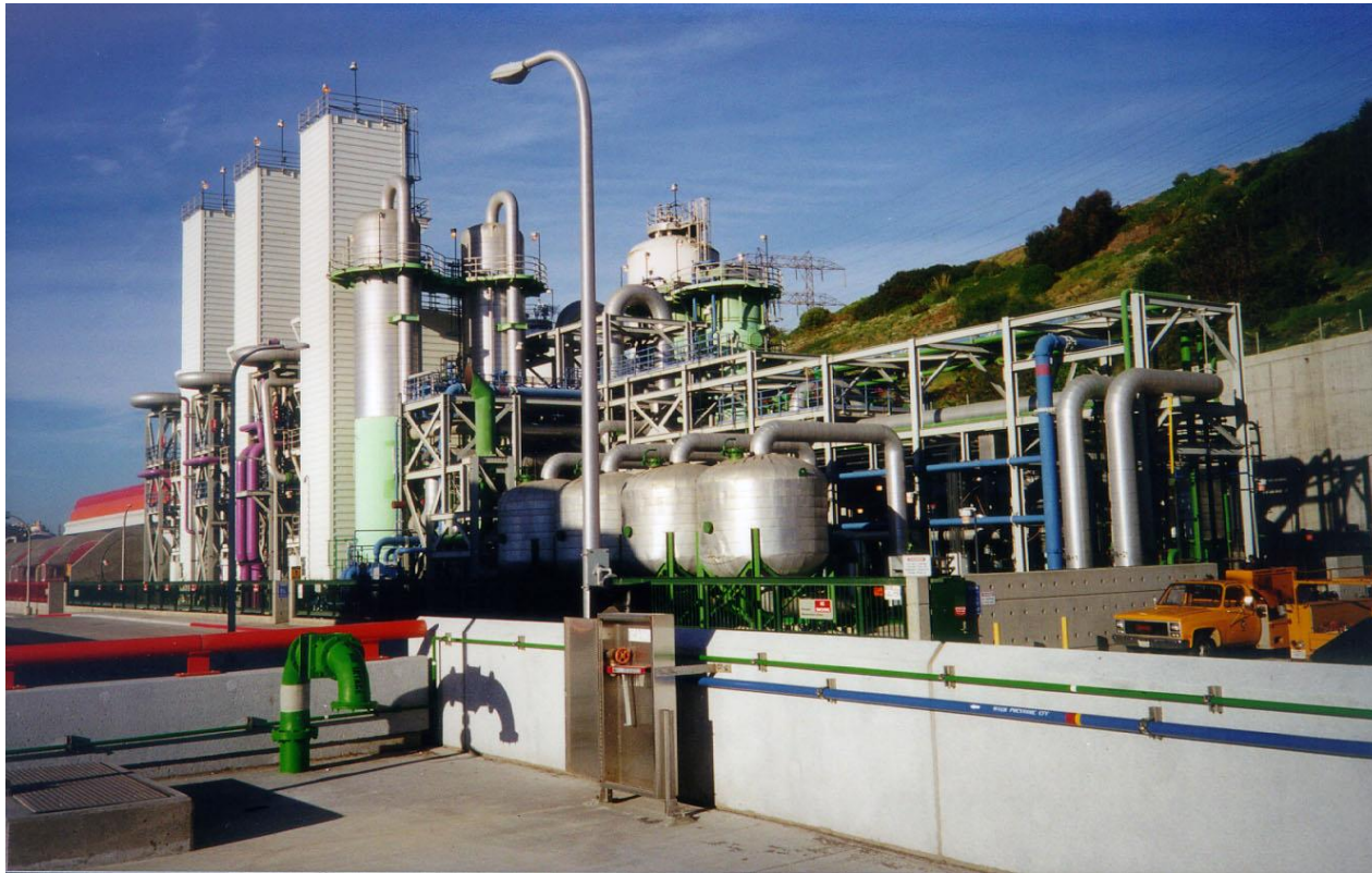
Cryogenic air separation facility, Hyperion, Playa del Rey, (CA)
