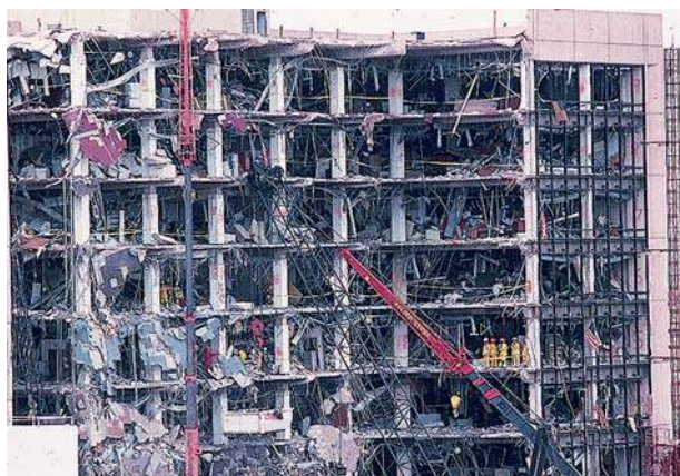
The Alfred P. Murrah building after a deadly explosion caused by an ammonium nitrate bomb.
