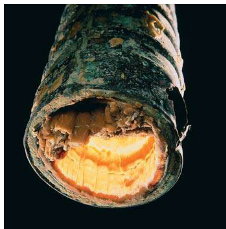
Boiler scale almost fills this hot-water pipe. The deposits consist mostly of \text{CaCO}_3 with some \text{MgCO}_3 .
